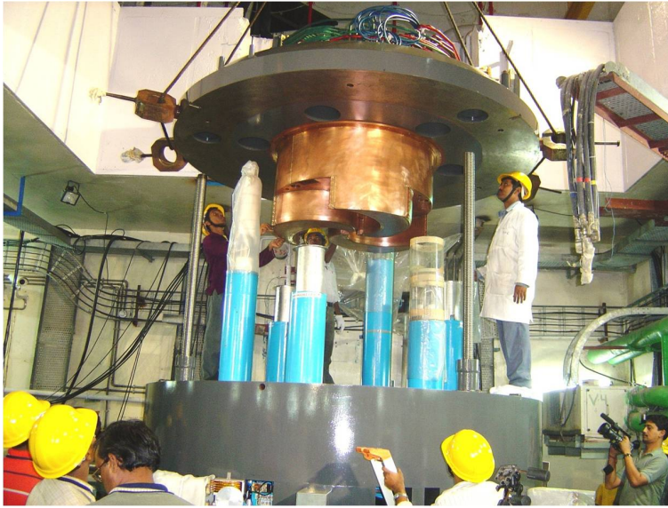
The upper half of magnet iron structure
